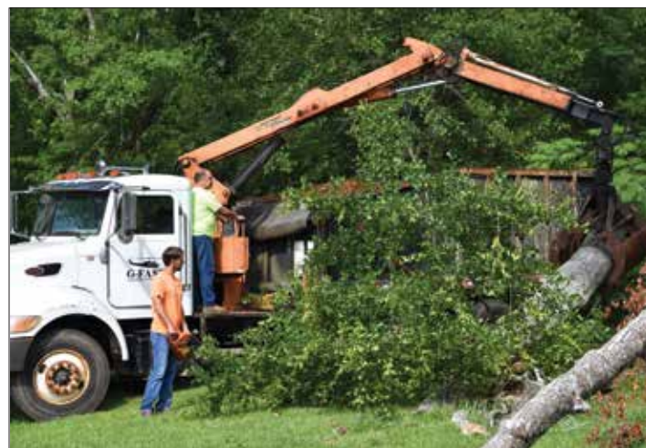
Del Loveless (on ground) and Richard Connell (on truck) cut down and clear away a tree for a local agency. G-FAST offered to remove the tree at no cost to the Jefferson County non-profit, saving them several hundred dollars.
